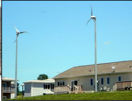
Net Metering Small Wind Energy Systems Winnebago, Nebraska.
